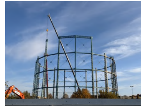
Demolition of the locally listed gasometer at Mitcham Gasworks – during a year when Merton Council unilaterally rewrote the site’s planning rules and there was minimal public engagement by tower blocks developer St William
